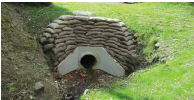
Rehabilitation work was undertaken on the inlet to the stormwater drain located on Butler Street Te Kuiti.
